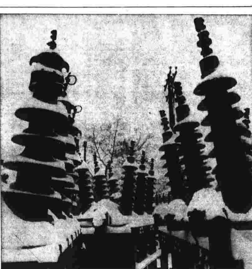
Weekend Snow Insulates Rockville Insulators Looking like some sort of futuristic Christmas trees, these insulators atop spare transformers in Rockville are "insulated" by the weekend snow. The area was covered by a white blanket five to eight inches deep yesterday — the season's first severe storm. (Herald Photo by Saternis.)
